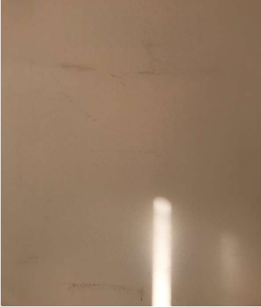
Scuff marks to wall
