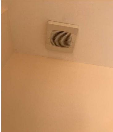
Dusty on inspection, advised tenant to clean to avoid breaking
